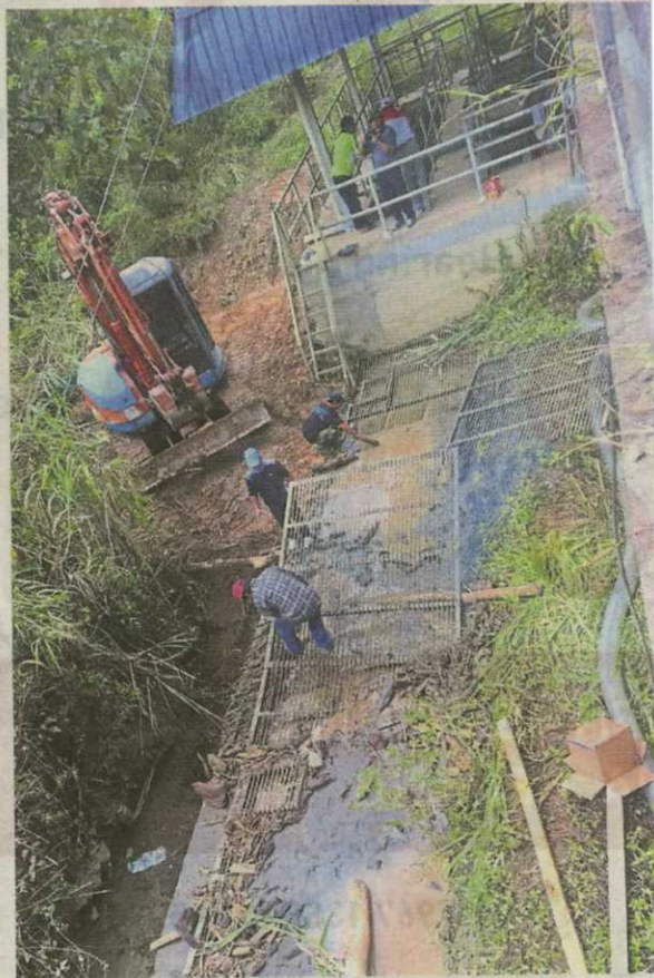
Plan B: Engineers and workers building an alternative water channel to the Kampung Bambang water intake point in Ranau.
