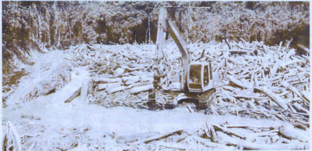
Work in progress: An excavator being used to clear the timber debris in Sungai Liwagu where the Ranau water treatment intake point is located.
