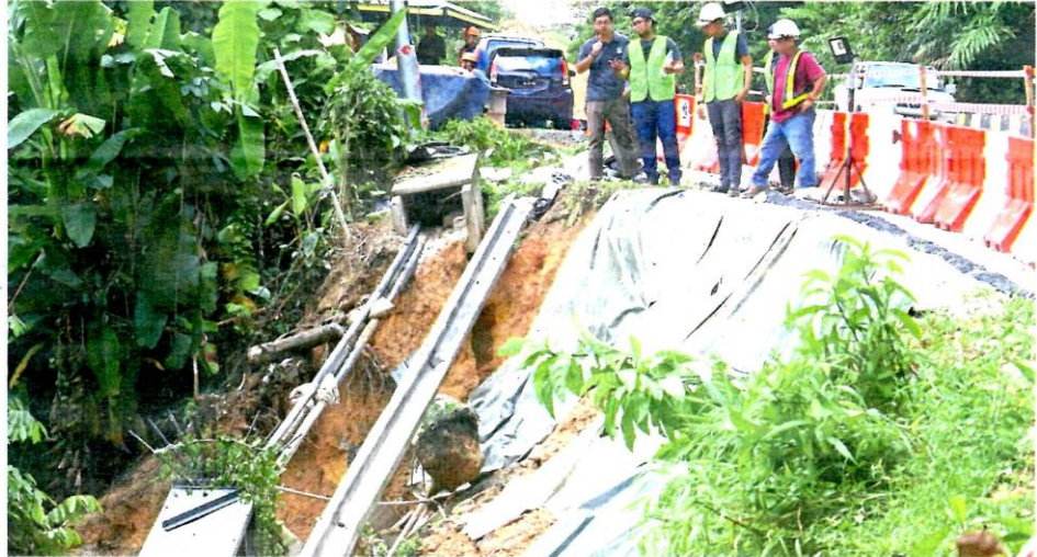
Dangerous: File photo of a landslide area along the hillside road of Jalan Paya Terubong, Penang, being worked on. Hill slopes and development do not go together, yet development in such sensitive areas continues.
